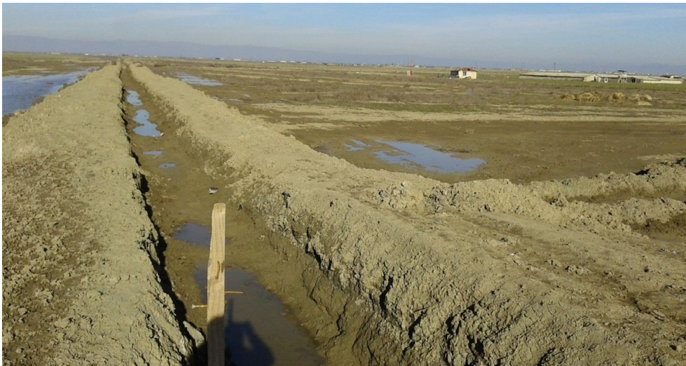
Figure 3. The actual state of the collector-drainage network
